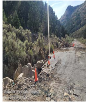
Photo 8 Middle fork road repair in progress, rock fill taken from flood debris
