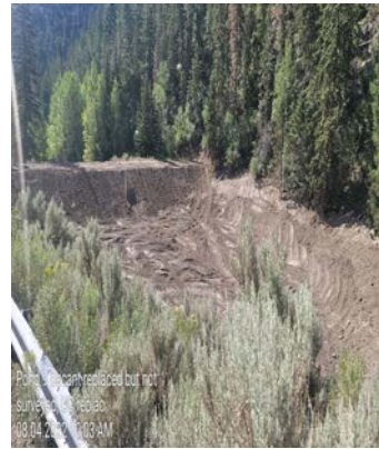
Photo 10 Pond 9 decant replaced but not surveyed or cut to height yet, 42in CMP UC replaced
