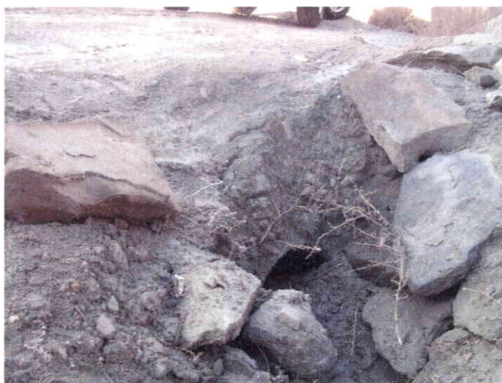
Photo 1. Partially blocked inlet to culvert in ditch DD-2a
