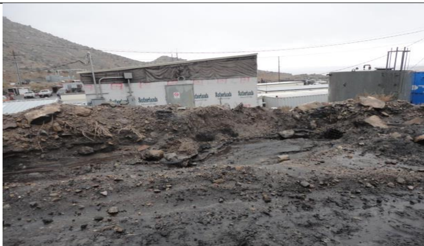
PHOTO 4 Diversion DD-3 Needs Clean out
