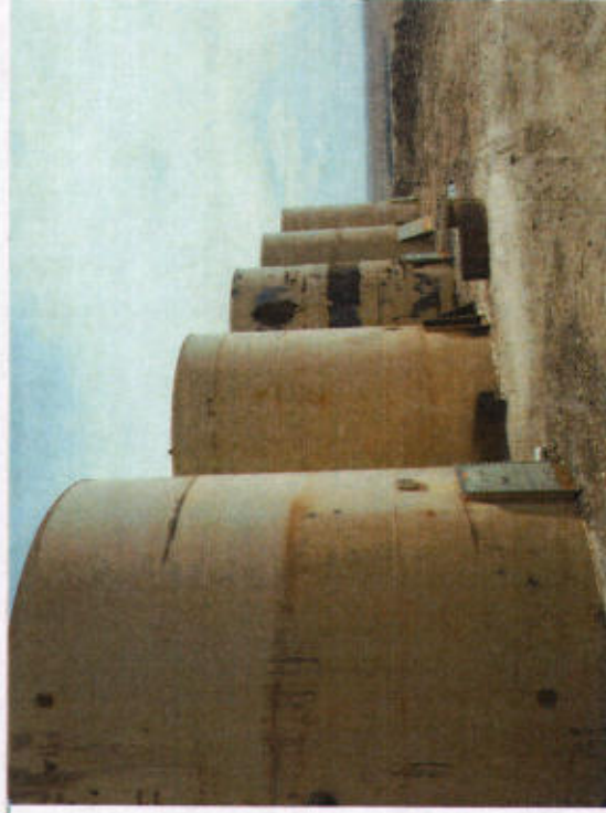
Berm around tank farm should be built up to hold 110% capacity of the largest tank.
