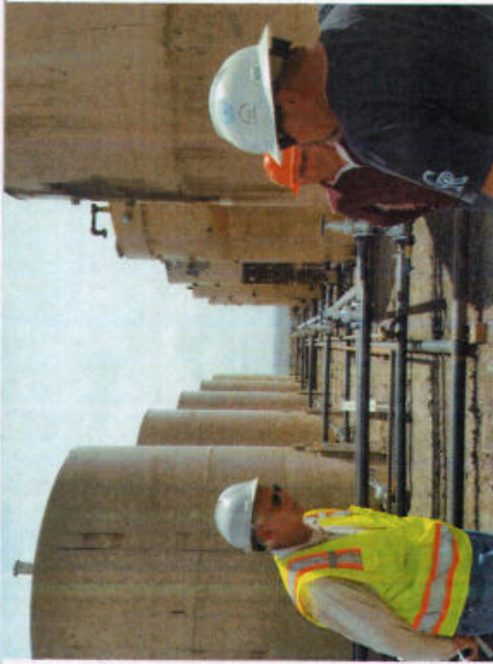
Photo 1. View of tank farm containing 15 storage tanks with crude oil and condensate products.
