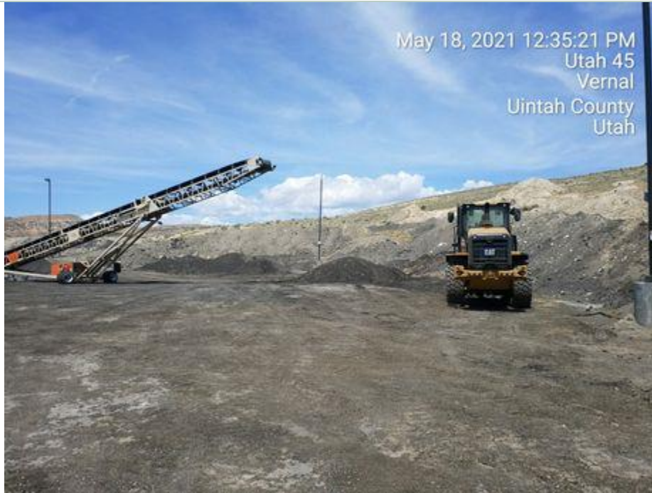
Latitude: 40.3373, Longitude: -109.48656 Small amount of ore was staged in front of the crusher.
